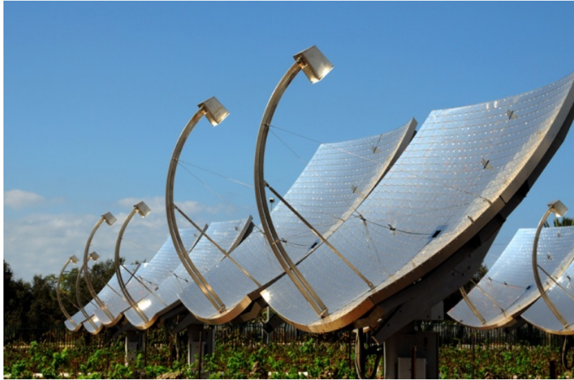
ZenithSolar Z20 CHP Solar Technology installation successfully operating at KibbutzYavne Israel since April 2009
